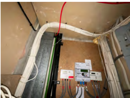
Electrical cupboard ground floor fire stopping required.
