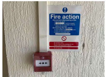
Fire action notice and call point adjacent to front entrance.
