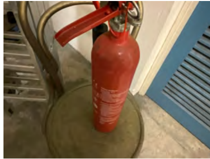
No service data sticker on lift motor room extinguisher.
