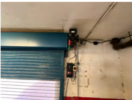
Manual override on car park shutter doors.
