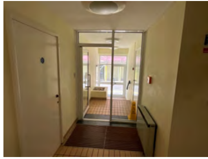
Further examples of a lack of fire exit signage.
