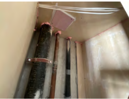
Poor fire stopping in mains water riser cupboard.
