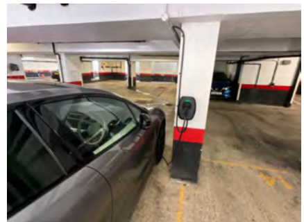
EV charger in car park area.
