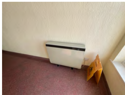
Storage heaters on a fused spur.
