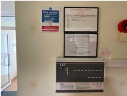
Fire alarm panel, zone chart and fire action notice.
