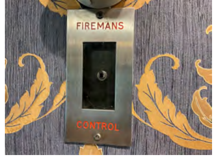
Fireman's control panel.
