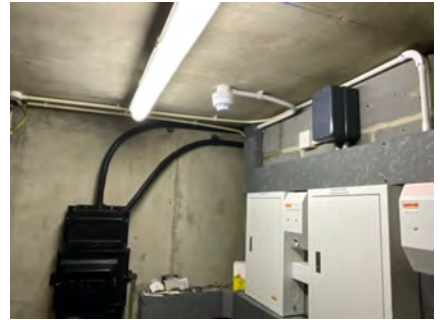
Detector in the electrical cupboard.
