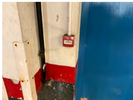
Call point adjacent to exit door.
