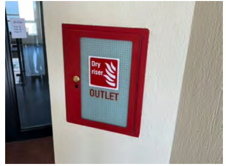
Dry riser outlet on all floors.
