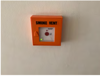
AOV operator adjacent to rear exit door.
