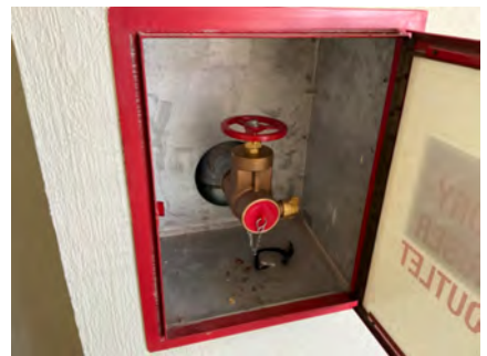
Dry riser 1st floor.
