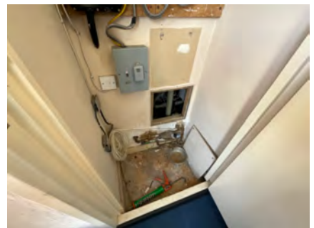
Sixth floor electrical cupboard.
