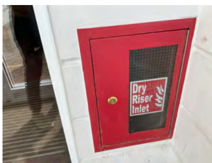
Dry riser adjacent to front entrance.
