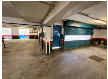
Lack of fire exit signage in car park area.
