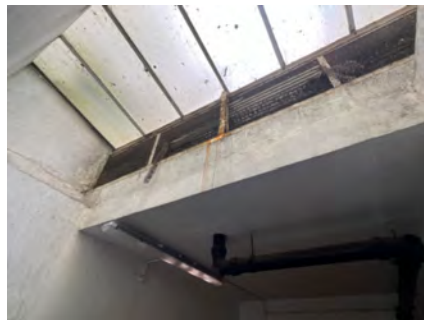
Ventilation in undercroft parking area.
