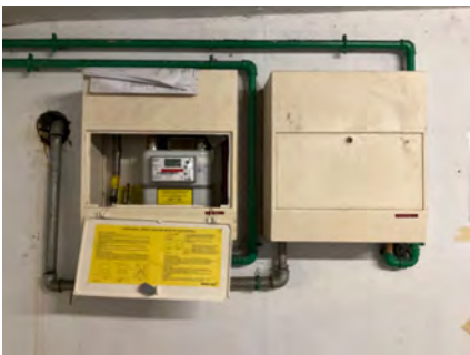
Gas meters in car park area.
